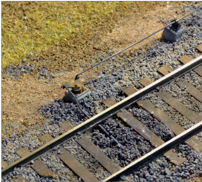
12. As the semaphore moves from the STOP position to the PROCEED position, the crank also moves. The crank lever for the derails also moves in relationship to the derail points.
