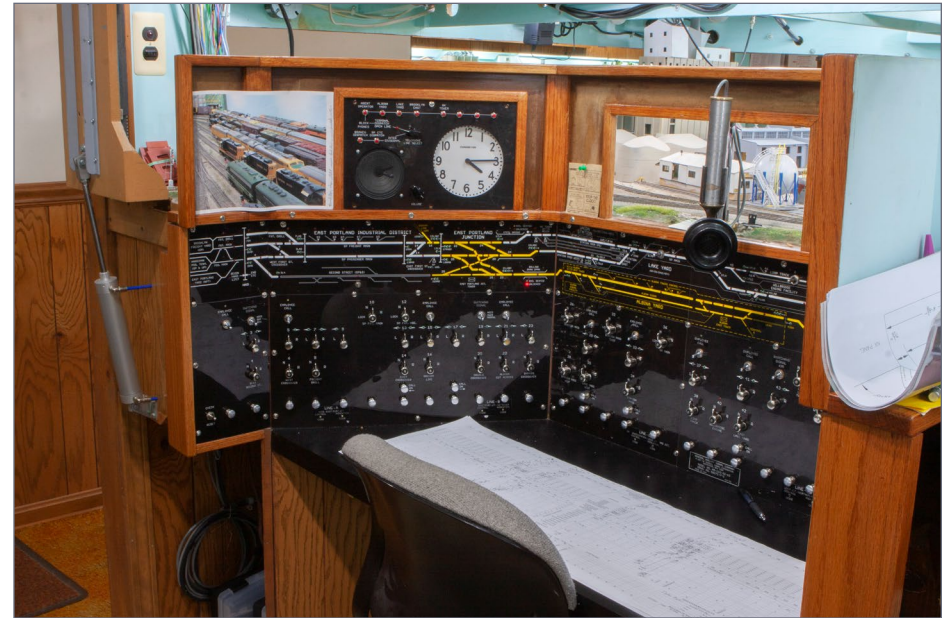
23. This CTC panel handles the Portland area GN and NP yards. On the prototype, the GRS panels are custom-built for each application and custom engraved.
